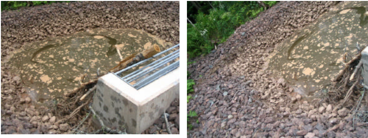
Figures 3 and 4: Drainage Structure off of Mapleton Park Path, Mapleton Brook located in background
